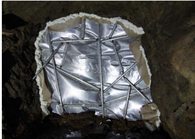
Figure 4: Quick-Erect Stopping System (QESS) in the crosscut Querschlag 60 to protect the construction site in the Markus Semmler gallery at the section Fleischer Morgengang in Schneeberg
