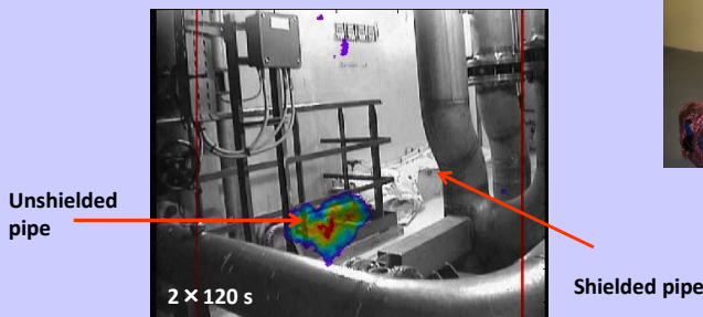
Partial shielding of a pipe
