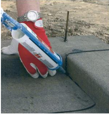
Figure 3. Installation of a strip of bitumen felt in the joint of foundation wall and floor slab according to the Finnish guidelines.
